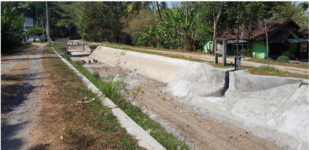
Figure 6.8: The closure of irrigation system has stopped water supply for farmlands and livestock
