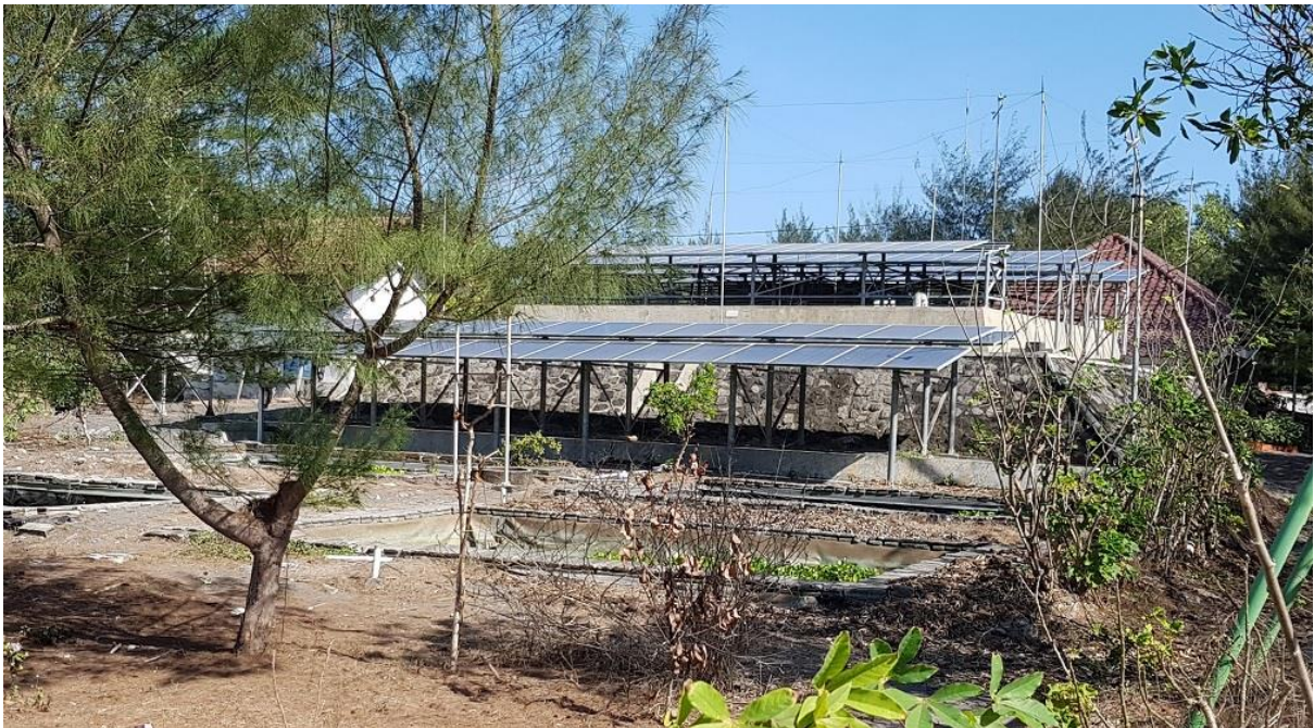
Figure 6.5: Solar Panels in PLTH Pantai Baru
