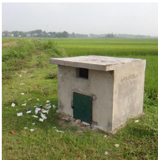
Figure 5-13: Concrete waste container in Ngoila system
