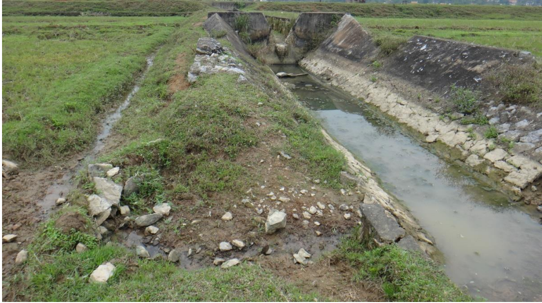
Figure 7-9: N6 secondary headwork degradation
