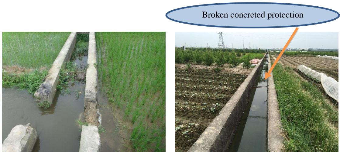
Figure 6-12: Canal broken (left picture) and canal protection lost (right picture)
