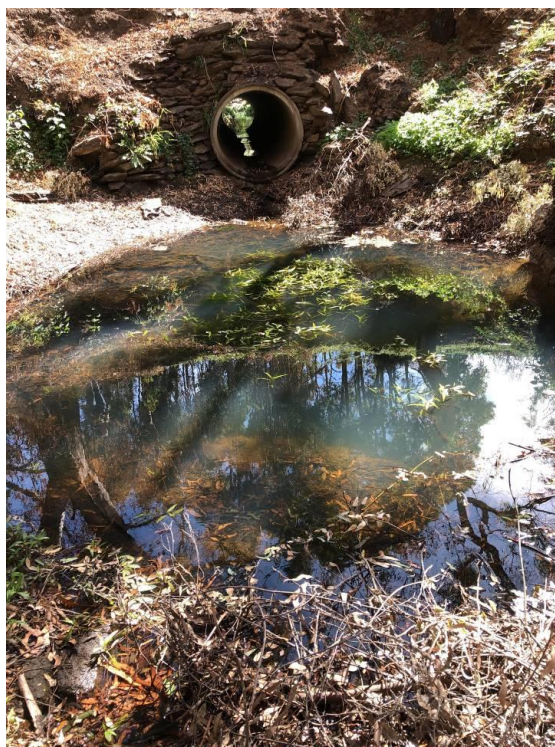
Figure 13: Ponding at 02 during CCWS01
