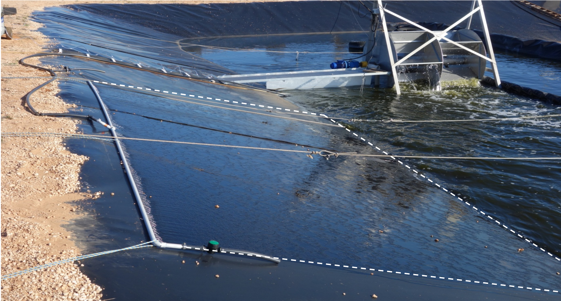
Plate 6.2: 20 m 2 IP (white rectangle) retrofitted to the Kingston on Murray (KoM) HRAP pond wall. IP was situated downstream of the paddlewheel and approximately 30 cm from the top of the pond lining.
