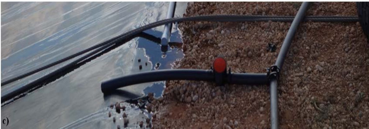
Plate 2.9: Components of the large scale IP system attached to the KoM pond wall. System was comprised of a) 25 mm grey electrical conduit, b) 25 mm black PVC flex tubing and c) ball-valves for flow throttling.
