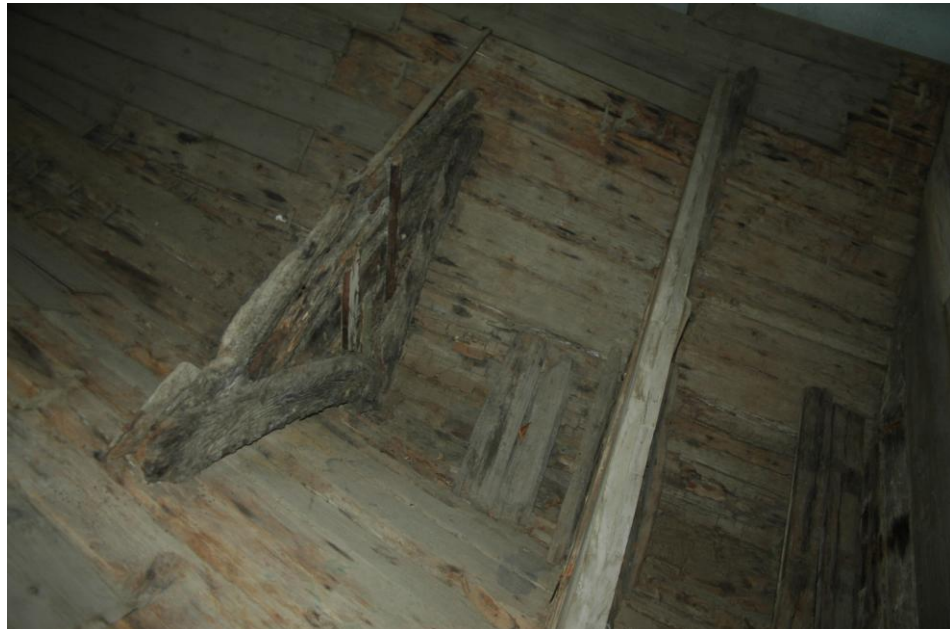
Figure 5-27 Top view of the Bulkhead No.1 that has original half-frames. Photo by author
