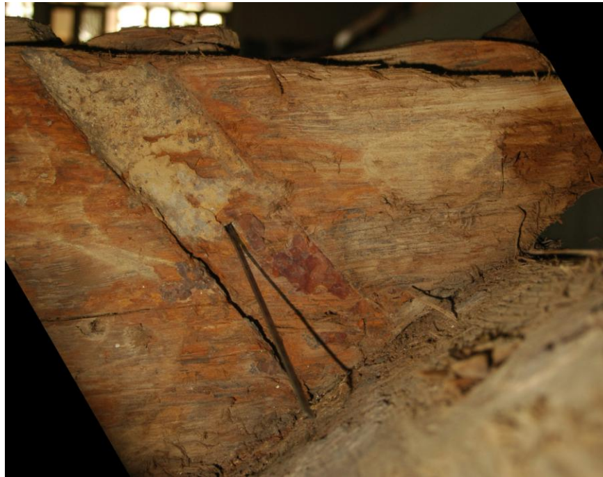
Figure 5-24 Bulkhead plank has the recess for a metal bracket to be attached where corrosion and a nail hole can be seen. The nail might have been driven diagonally upward.
