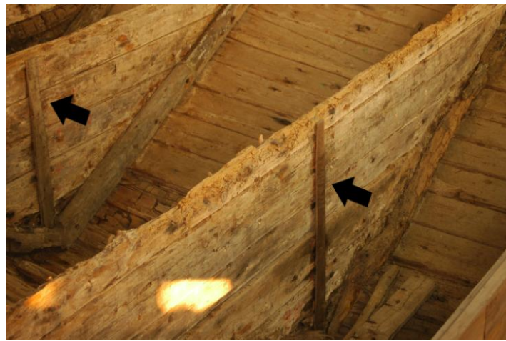
Figure 5-20 Wooden strips standing in the Bulkhead No. 10 and No.11 representing the reconstruction of the original bulkhead stiffeners. Photo by author
