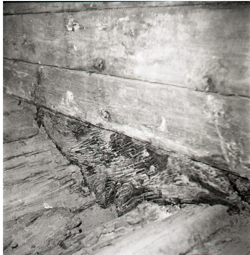
Figure 5-22 Photograph showing the degraded bottom bulkhead plank. Courtesy of Museum of Overseas Communication History
