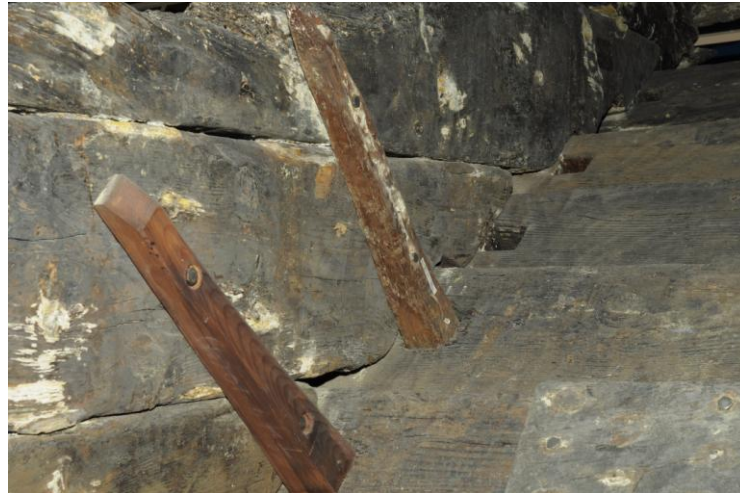
Figure 6-27 Wooden brackets fastened into the surface of the bulkhead planks. Photo by author
