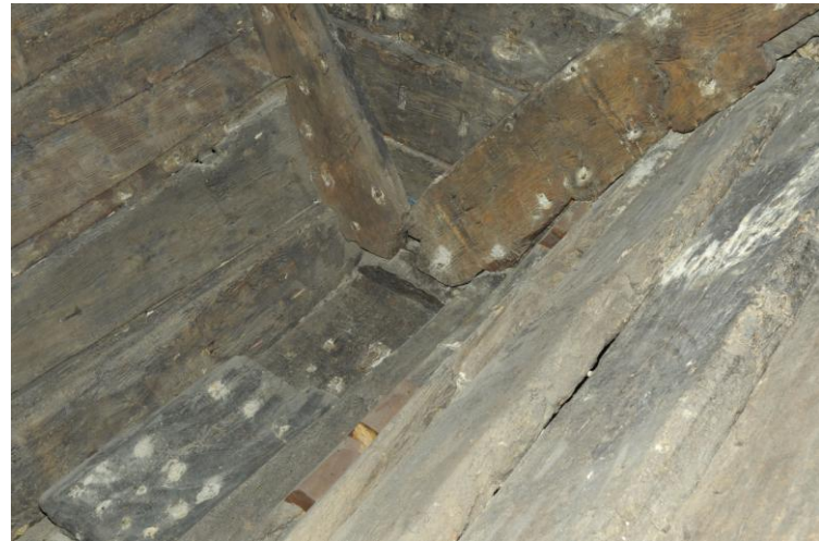
Figure 6-24 Limber cut in the bottom end of the frame. Photo by author
