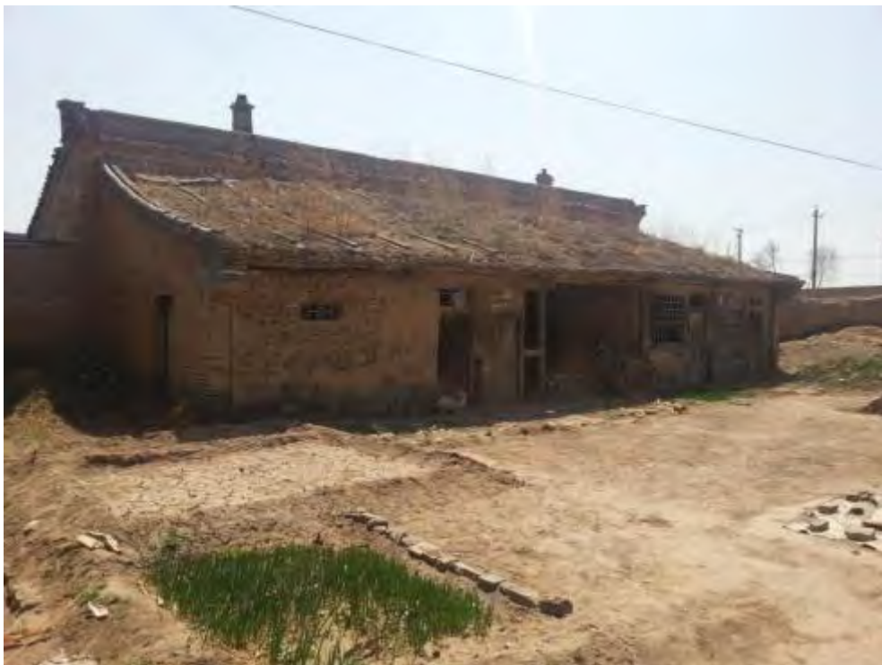
Figure 18. Dilapidated ancient residential courtyard
