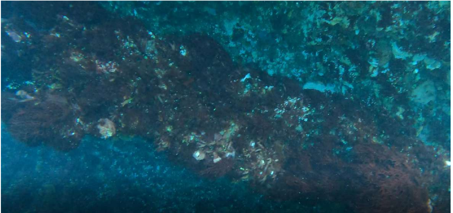
1G.22. ADM1-020 rudder trunk angled support frame heavily deteriorated underneath main 'A' frame (2022-01-12, P. Kermeen)
