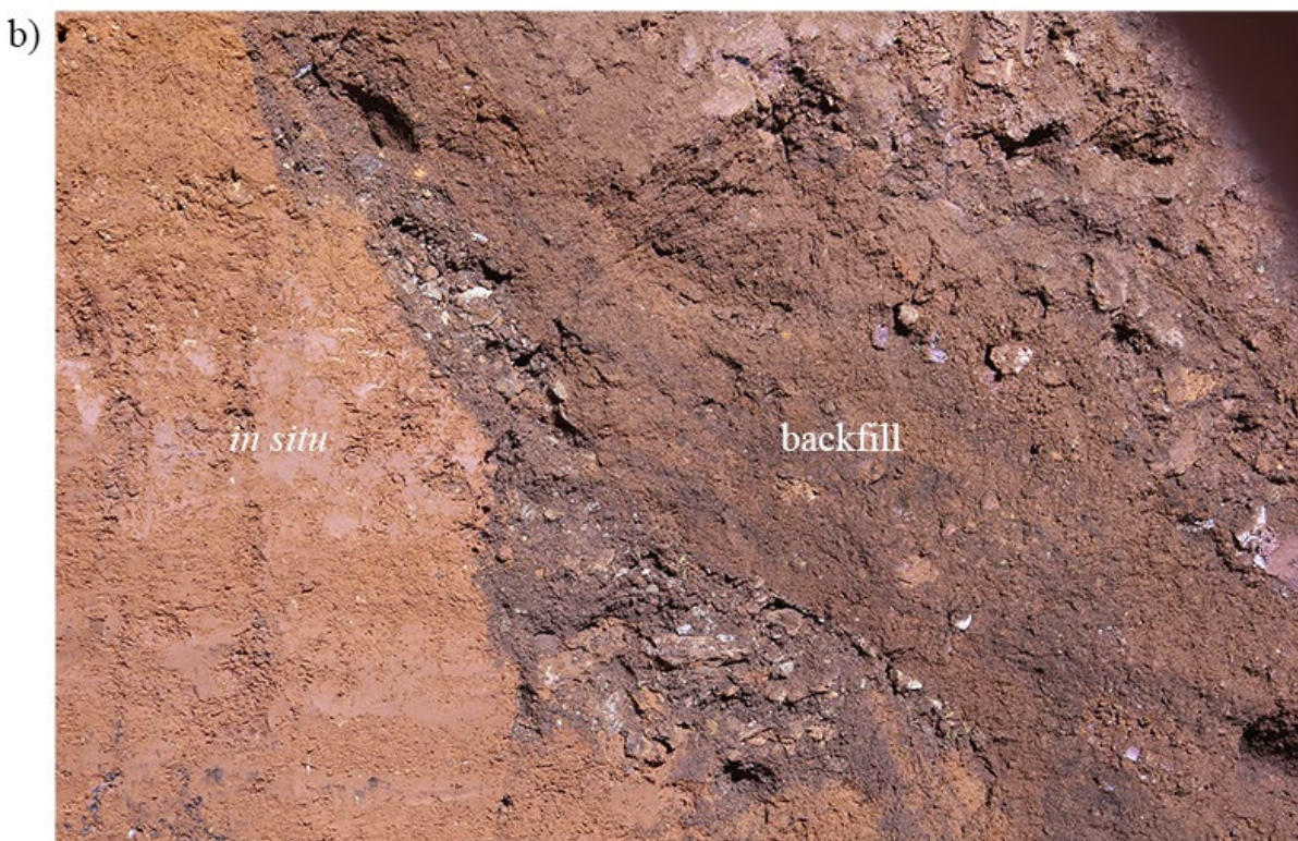
Figure 3.6. East wall of excavation showing a) boundaries between the in situ sediment layers on the left and the disturbed and backfill on the right; b) easily defined boundary between in situ sediment on left and backfill on right.
