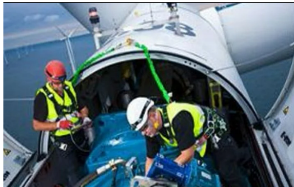
Fig10:Wind turbine maintenance
