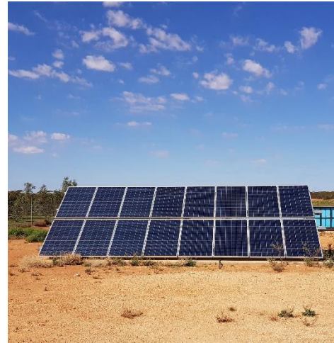
Plate 2.4 Solar panels providing electricity to HRAP at KOM
