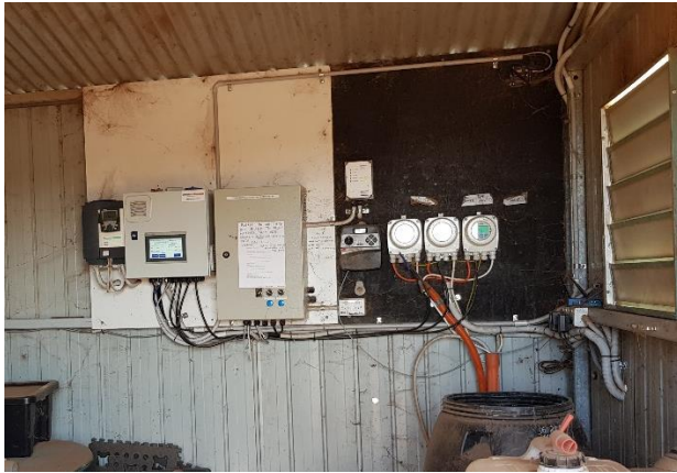
Plate 2.3 Control panels in shed
