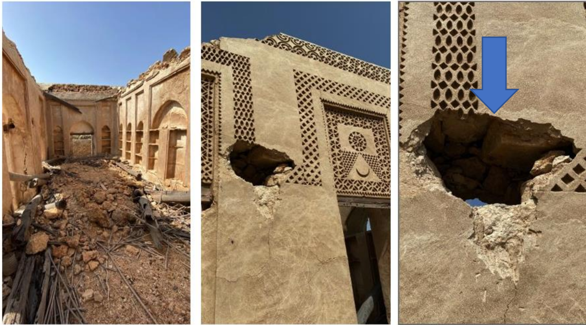
Figure 13: Turkish house with holes and no roof (Photograph: A. Refaei).
