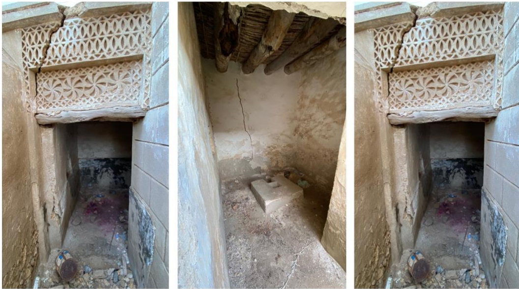
Figure 11: Back of Hussein Al-Rifai house: damage to internal features and conservation problems (Photograph: A. Refaei).
