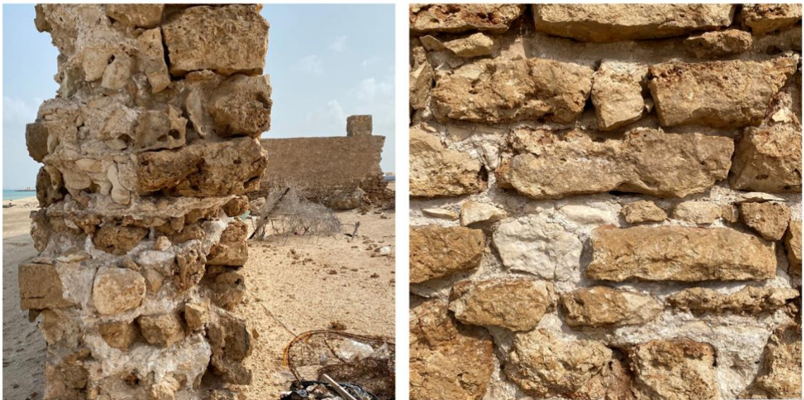
Figure 6: A wall of the German house, showing its building materials (Photograph: A. Refaei).
