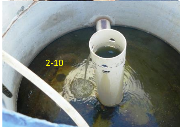
Plates 2-9 & 2-10 HRAP - Sampling directly from the inlet splitter box as the wastewater is flowing; and from the stand-pipe in the outlet control pipe.
