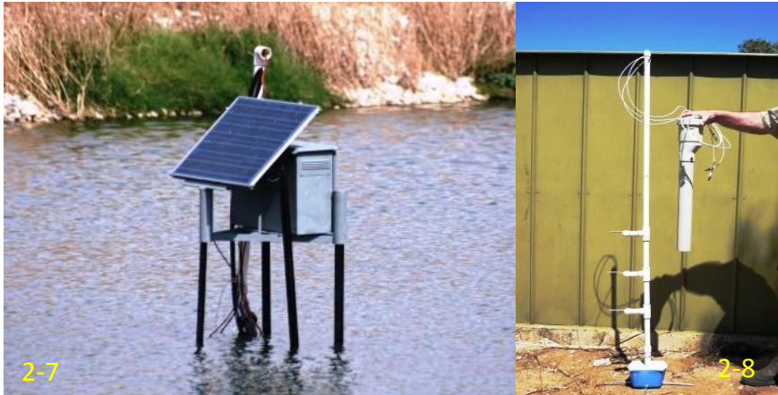
Plates 2-7 & 2-8. 2-7 Installed solar powered DO, pH and temperature monitoring box in mid-pond position. 2-8 Thermistor chain before installation mid-pond
