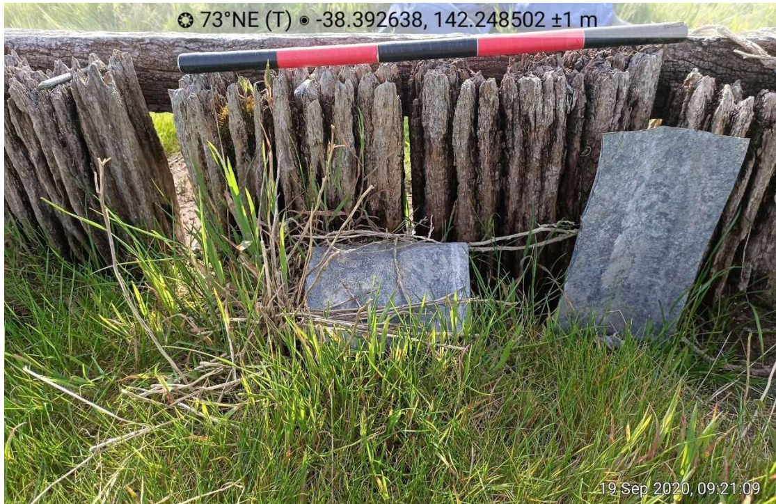
Figure 32: Inside of north wall, galvanised sheet metal covering exposed gaps in timber, holding earth in.
