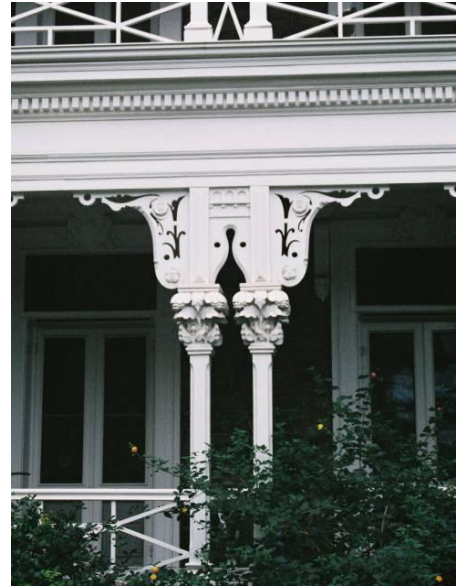
Figure 5.23 Parramatta Villa . Elaborately carved timber bracket. Photo: R. M. Stone, November, 2007
