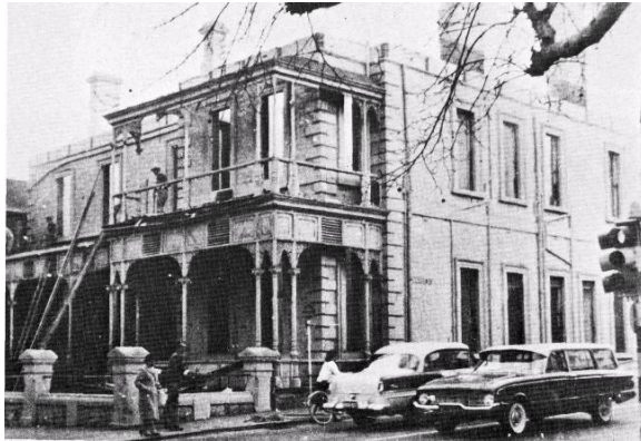
Figure 7.5 Demolition of Tavistock House , part of the widening of Frome Road, Adelaide. Source: Burden, 1983:33.
