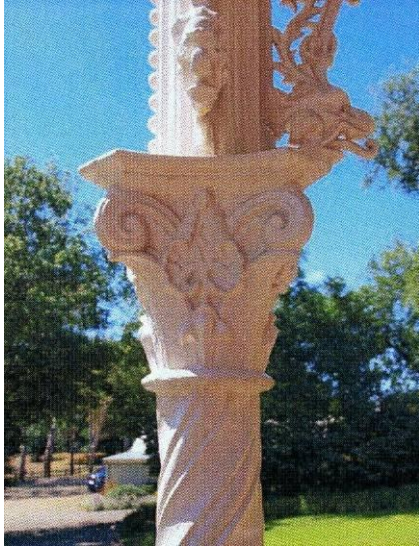
Figure 3.4 Dalintober , cast iron verandah post with dragon head. Source: Raine & Horne sale brochure, 2009
