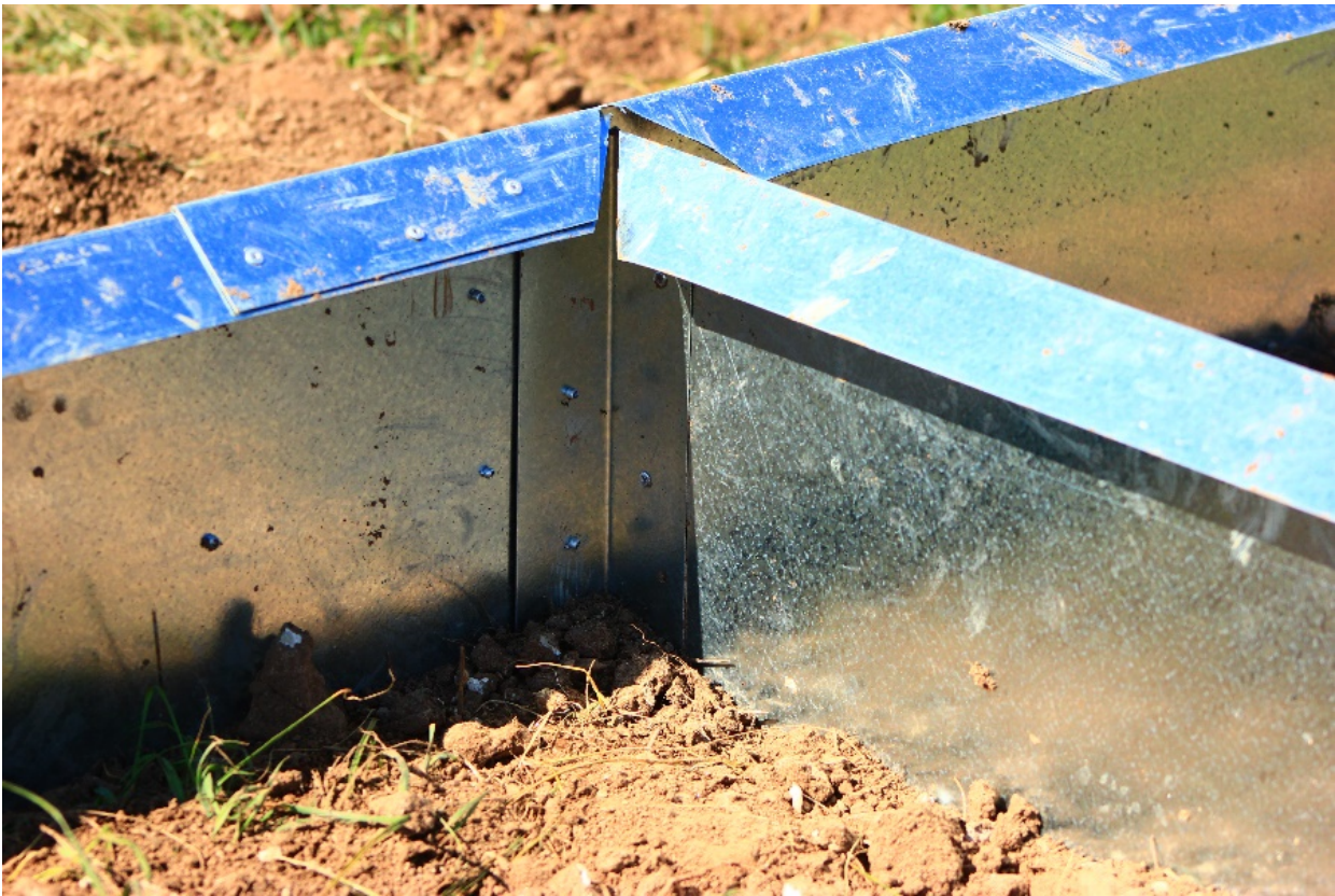
Enclosure wall made of galvanised steel with an inward facing lip
