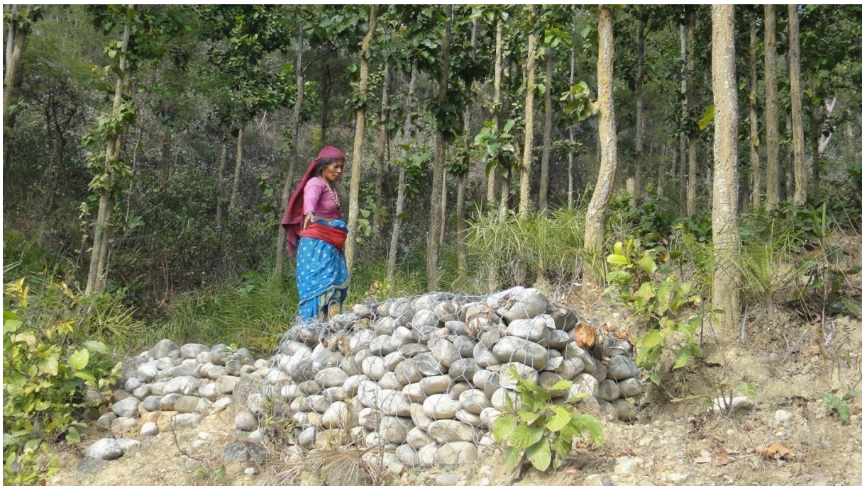
Figure 23: Construction of stone and gabion check dams as part of climate change risk-reduction activities in Bangesaal VDC (Photo Credit: Author)
