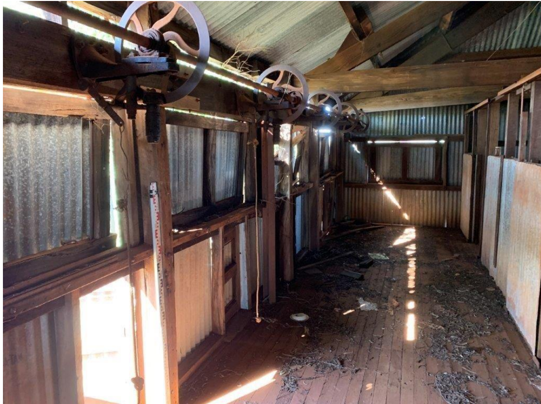
Figure 45: Shearing floor with overhead shaft drive for shears (photograph: Bart King)
