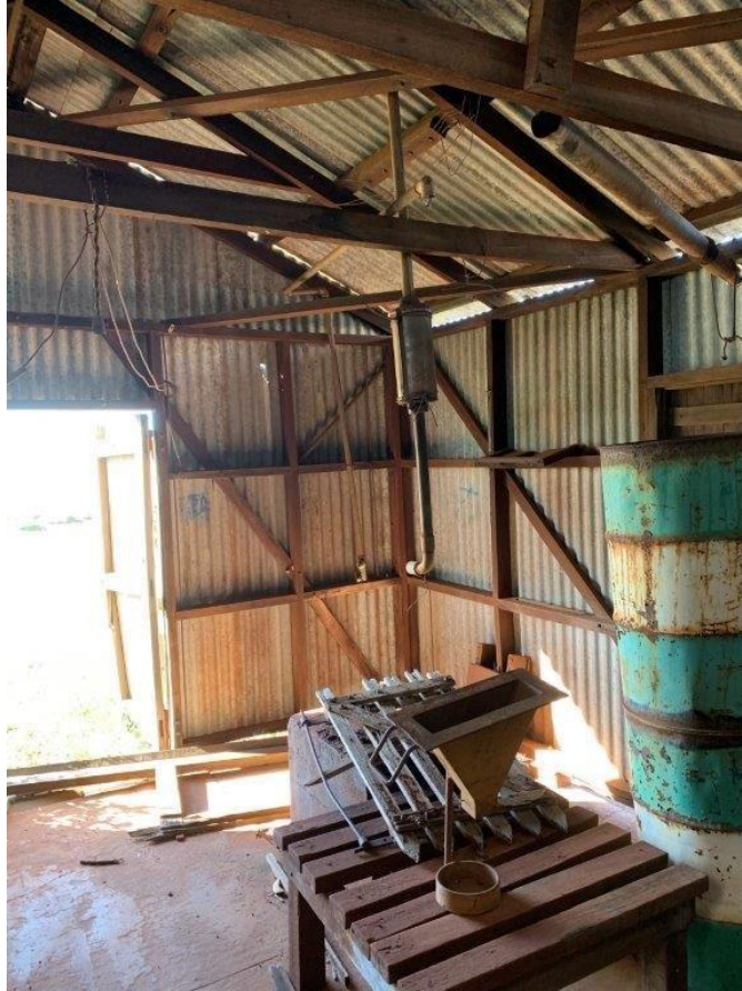
Figure 46: Engine room showing slab that engine was mounted on and exhaust still in place. (Photograph: Bart King)
