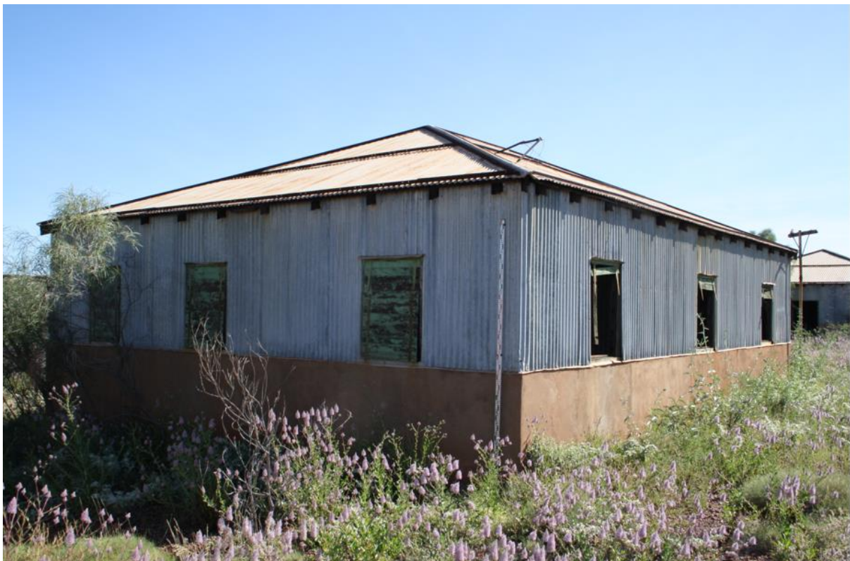
Figure 25: Balmoral dining hall eastern side. 1.2m concrete wall and roof layout. (Photograph: Bart King)
