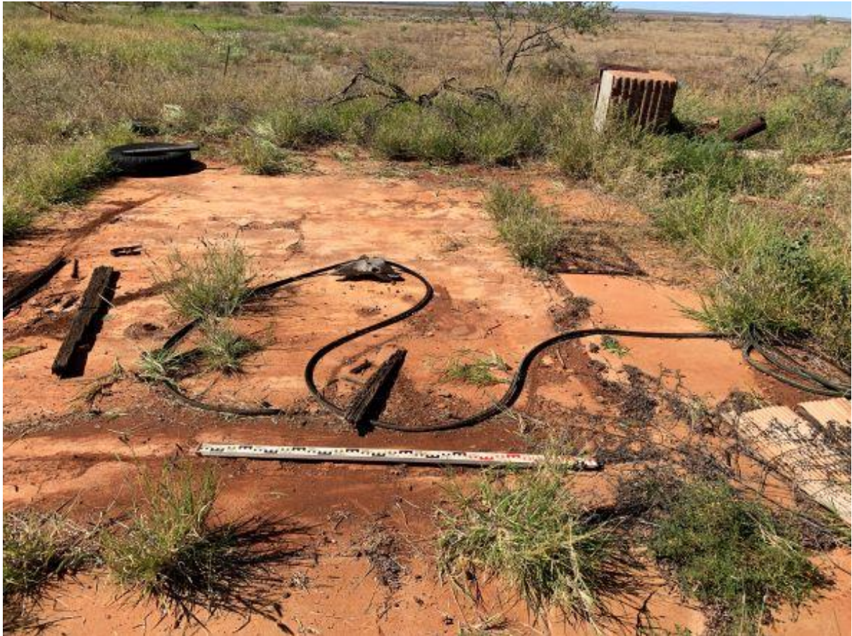
Figure 36: Concrete slab of Indigenous house with timber, metal fasteners and corrugated iron. (Photograph: Bart King)
