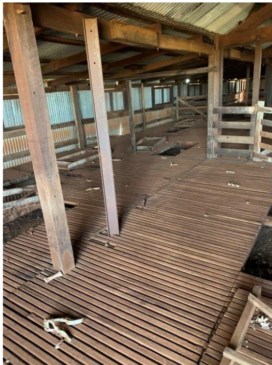
Figure 44: Catching pen area with removable floor panels (photograph: Bart King)
