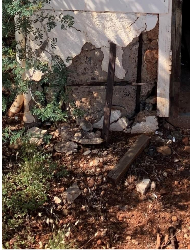
Figure 18: Concrete section of walls made up of reinforced concrete and render. (Photograph: Bart King)
