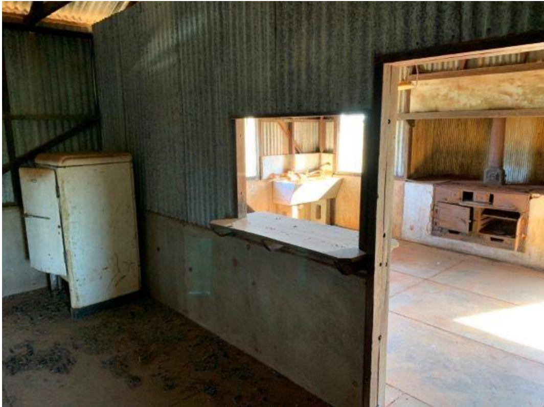
Figure 22: Servery in wall and wood fired, cast iron oven. (Photograph: Bart King)
