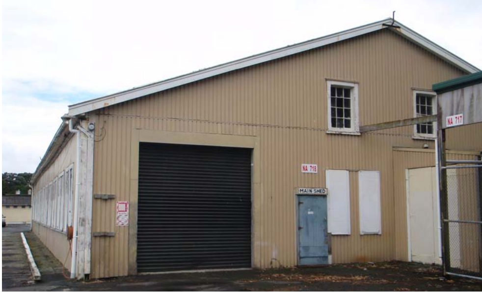
Figure 29. The former connecting-up shed at Torpedo Bay as it appeared in November 2008, showing wood-framed/corrugated sheet metal construction typical of most of the submarine mining station's 1886- and 1899-era standing buildings.
