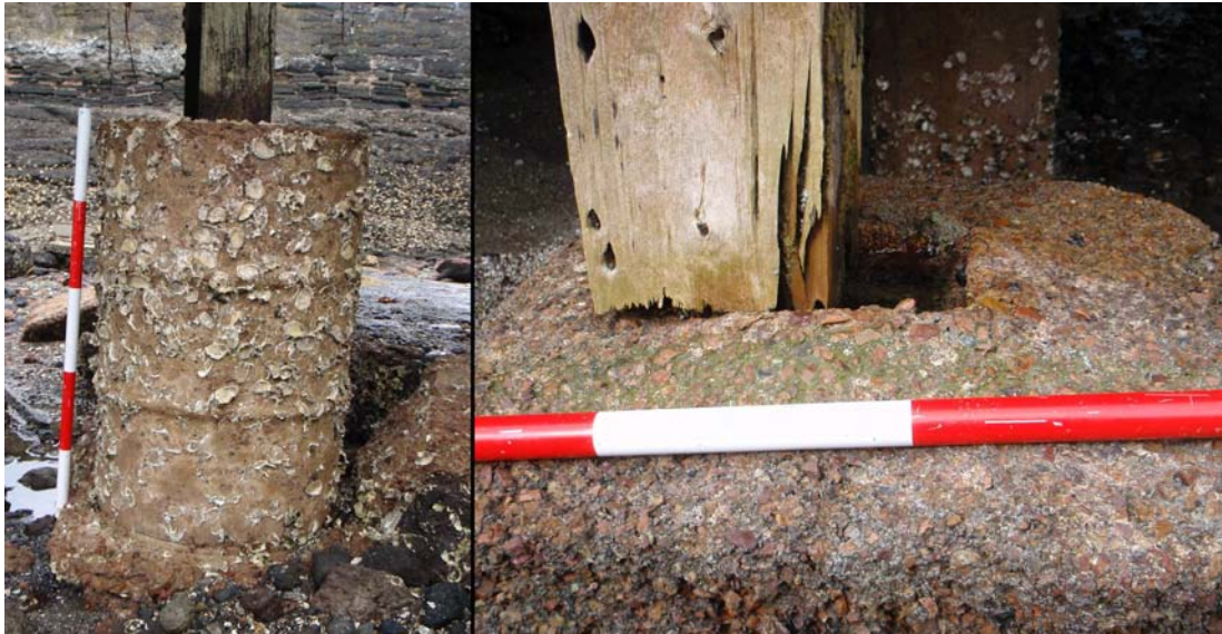
Figure 32. Left , concrete boat shed pile footer, as it appeared in November 2008, showing impression of steel 50-gallon drum ‘mould’; right , broken and partially dislodged wooden boat shed pile. Note deteriorated condition of wooden pile in the latter photograph. Scales in 20-centimetre increments.
