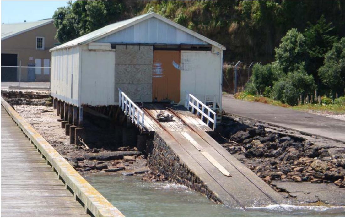
Figure 31. The second boat shed and slipway constructed for the Torpedo Bay Submarine Mining Station, as it appeared in November 2008. Note heavy corrosion along the base of the shed's corrugated metal walls, the use of metal sheeting and plywood to seal the windows and front door, and the presence of rubbish and other debris on the slipway.
