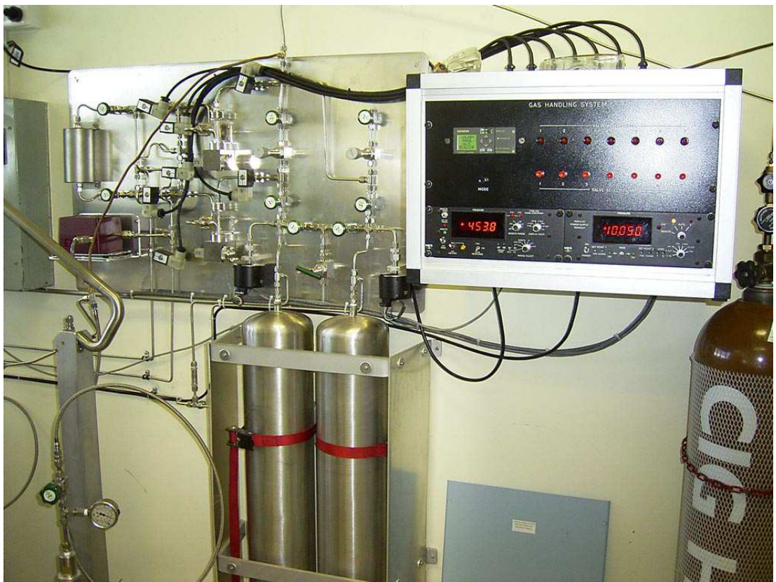
Figure 2.2.4: A Photograph of the present gas handling system.
