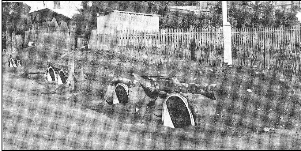
Figure 7-21: 36 in. x 8 ft pipes at Unley School awaiting installation of blast walls ( Hume Pipe News 1942: 4)
