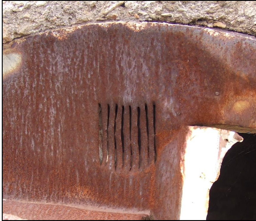
Figure 7-37: Detail of air vent, Chapman Type V shelter (Wimmer 2010)
