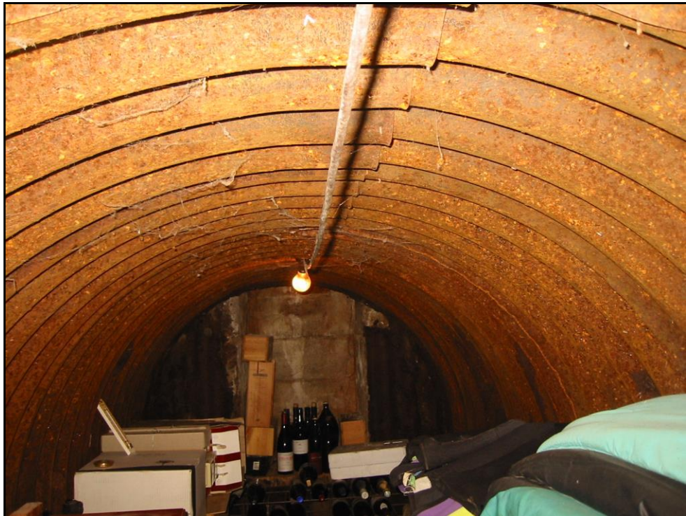
Figure 7-17: Inside the Hazelwood Park Type III shelter facing the rear escape hatch (Wimmer 2010)
