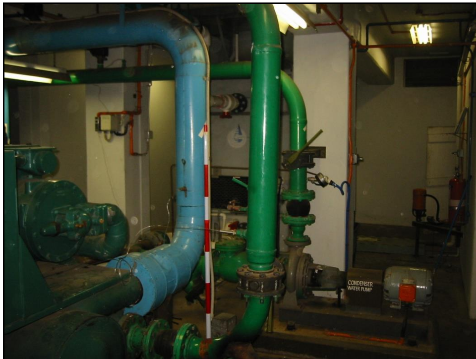
Figure 10-7: Plant room, Oxford Terrace Type V shelter (Wimmer 2010)
