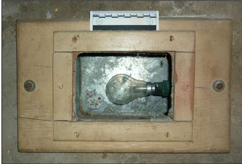
Figure 7-39: Emergency light, Jackson Type V shelter (Wimmer 2012)
