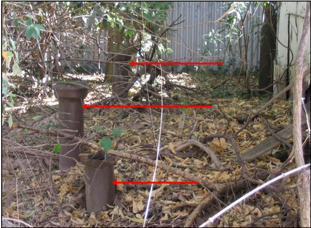
Figure 8-4: Three breather pipes (arrowed) above the Williamson shelter, Prospect (Prospect Local History Group 2009)
