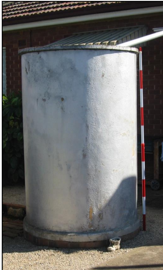
Figure 10-3: A concrete pipe rainwater tank, Kilburn, SA (Wimmer 2012)
