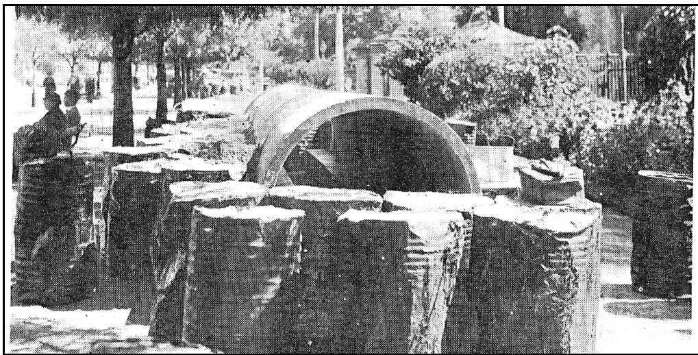
Figure 7-20: Fully accessorised: 48 in. x 8 ft pipes installed on North Terrace with sand filled bitumen drums being used in lieu of sandbags ( Hume Pipe News 1942: 5)
