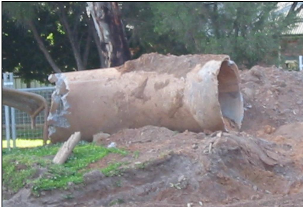
Figure 10-1: Excavated playground pipe, Mitcham Primary School September 2009 (Wimmer 2009)
