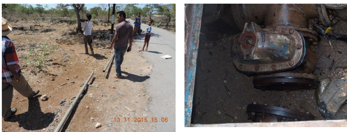
Figure 40: Networks that were discontinued and disconnected (photos by author)
