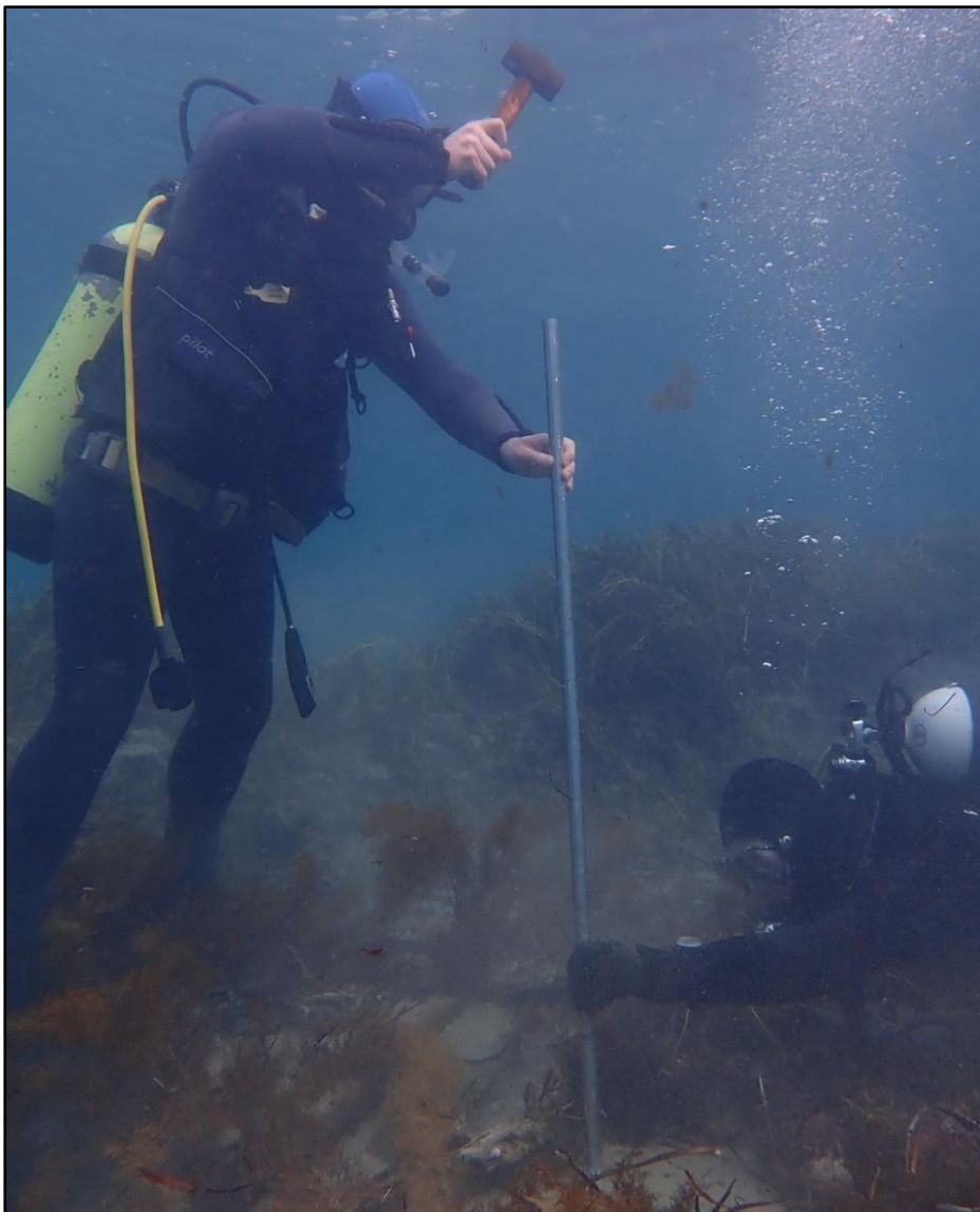
Figure 3.16. Kevin Jones and Timothy Zapor installing a sediment monitoring station (Photograph by Irini Malliaros, June 24, 2019)
