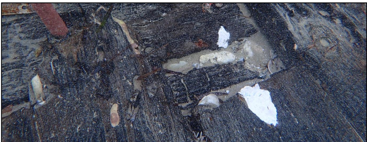
Figure 3.5. Aqua putty (white) inserted into timber sample locations (Photograph by Timothy Zapor, June 24, 2019)
