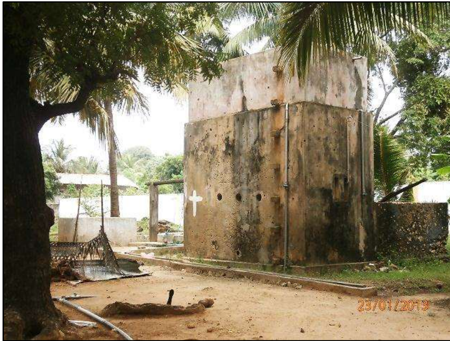
Figure 4.6 This overhead tank supplies water for drinking and cooking purposes for nearly 300 children. It has no cover to protect it from being contaminated. The management has ignored the danger to health and hygiene of the charges
