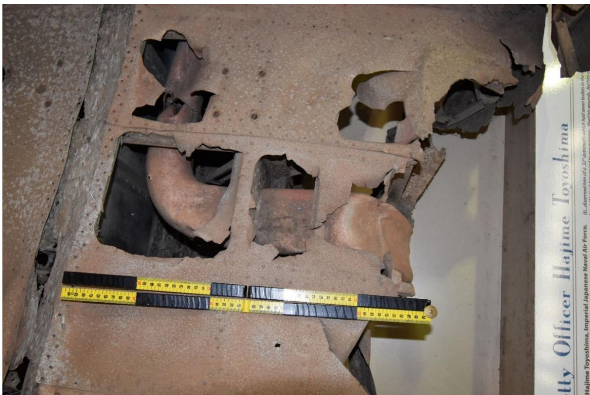
Figure 4.13. A fresh air ventilation tube to the cockpit in the starboard wing (the front is on the right of the figure) (Photograph: Author, 2 December 2021).
