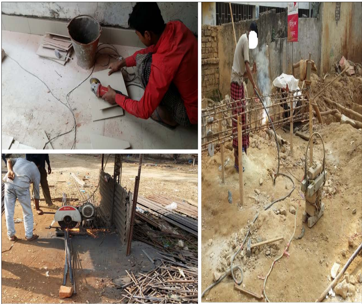
Figure 4.5: Workers operating electric machines without wearing PPE
