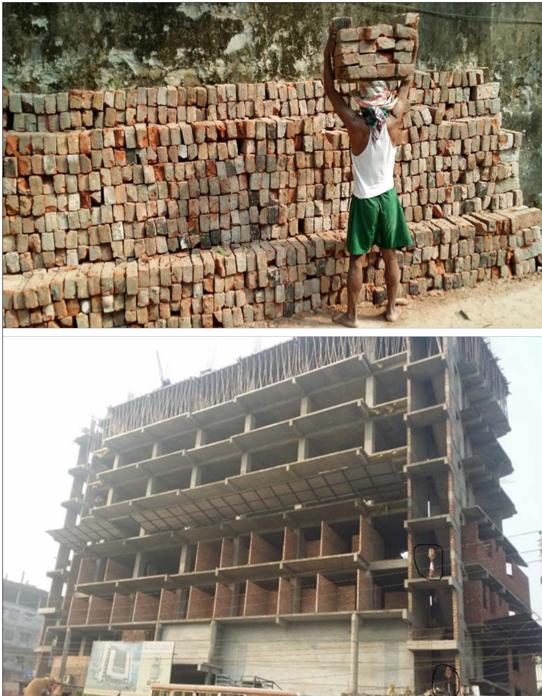
Figure 4.3: Workers lifting bricks, to the 6 th floor of a building, for the whole day
