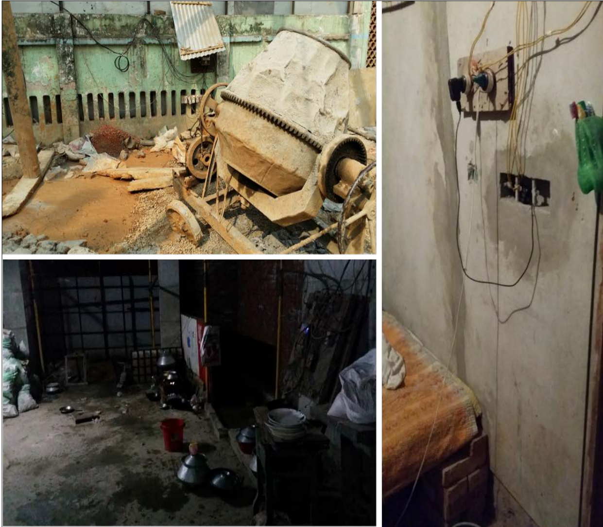
Figure 4.9: Unorganised power cables and switchboards in dining space and sleeping room
