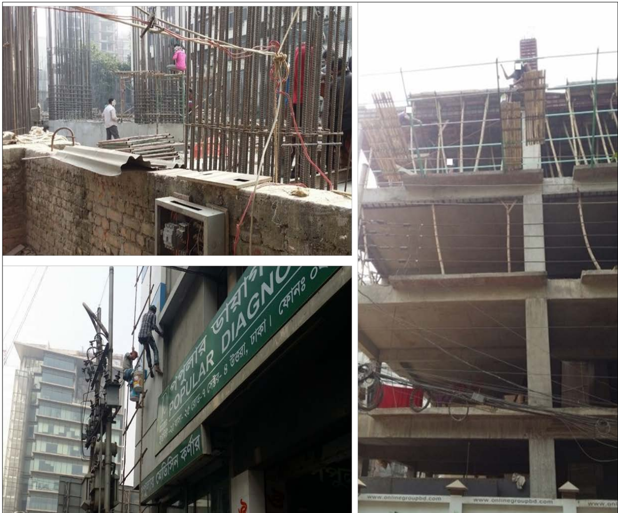
Figure 4.8: Workers working near electric switchboard, transformer and overhead power line
