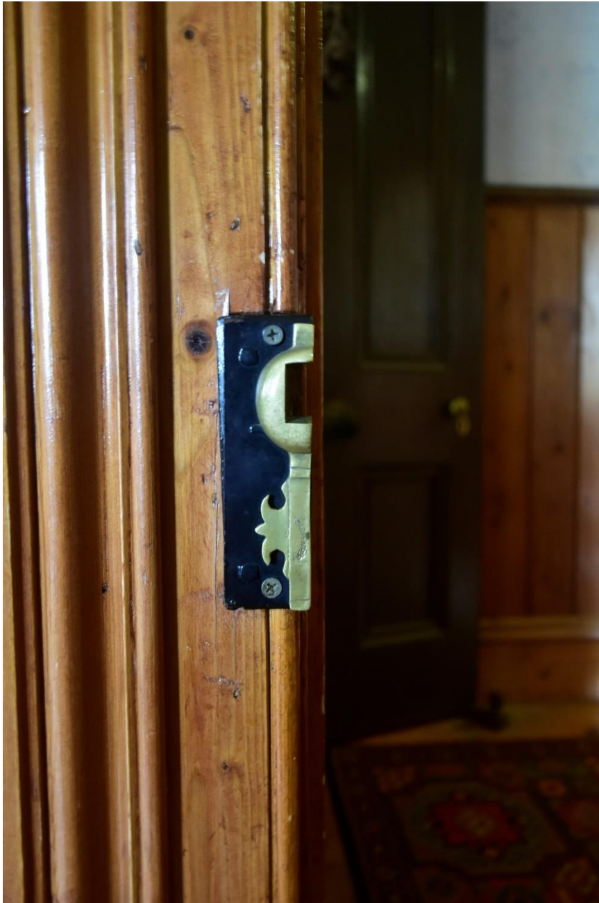
Figure 6.6.4 An example of the newer elaborate rim lock in Amess House. Aside from the technological advancement of the mechanism fitting into the wood of the doorframe, the flamboyant gold key design is a statement of wealth and status in Amess House (Rünzi 2021).
