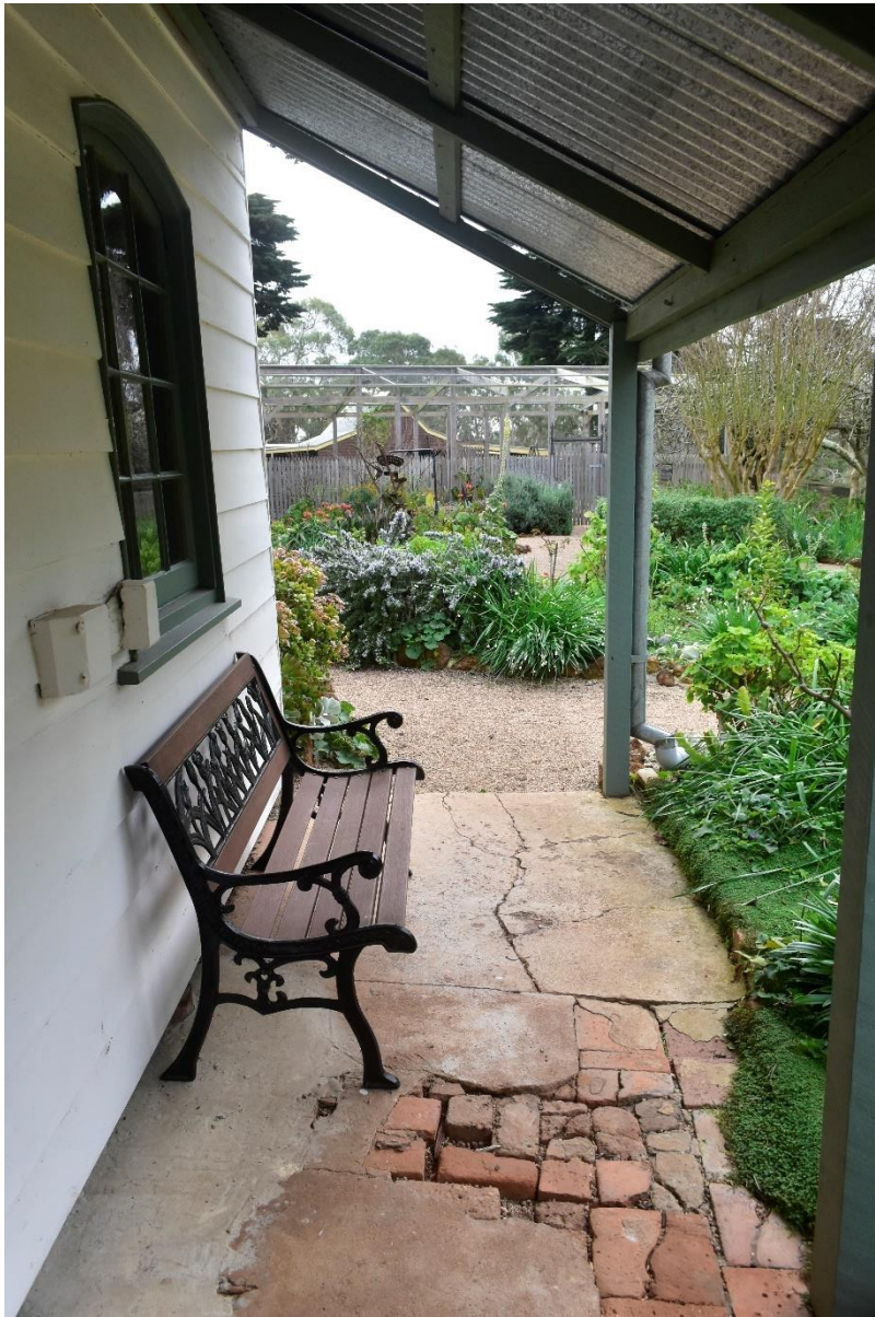
Figure 5.2.1.4 The front porch of the northern Rogers' Cottage. Note the layers of flooring, including larger square bricks, irregular rectangular and broken bricks, and a partially removed overlay of a concrete like material (Rünzi 2021).
