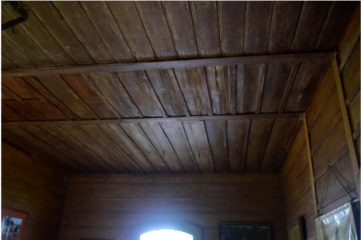
Figure 5.2.1.2 Details of the joinery on the ceiling of the northern Rogers' Cottage (Rünzi 2021).
