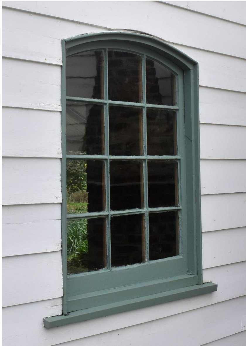
Figure 6.5.4 The windows of the northern Rogers' Cottage, arched in shape, unable to be opened, and containing no window furnishings (Rünzi 2021).
