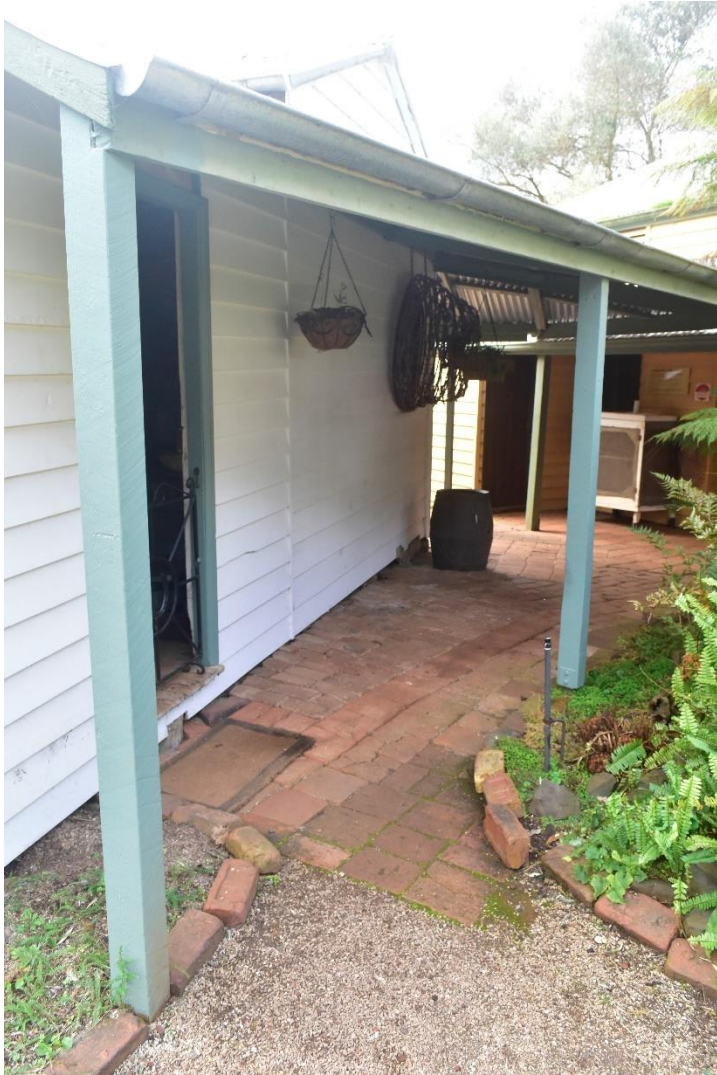
Figure 5.1.1.2 An east-facing view of the southern Rogers' Cottage. The door visible on at left leads into the small storeroom. The yellow walled building in the background is Amess House (Rünzi 2021).
