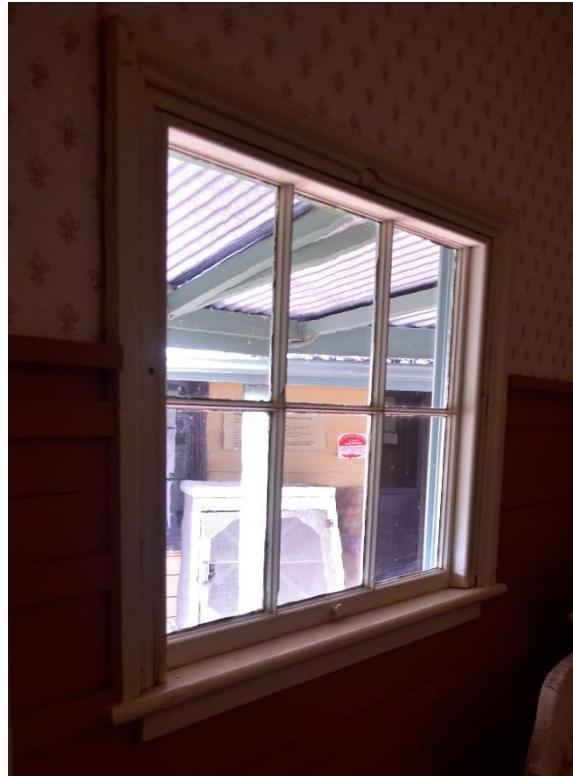
Figure 6.5.5 The windows of the southern Rogers' Cottage, flat arched in shape and with the ability to be opened (Rünzi 2021).
