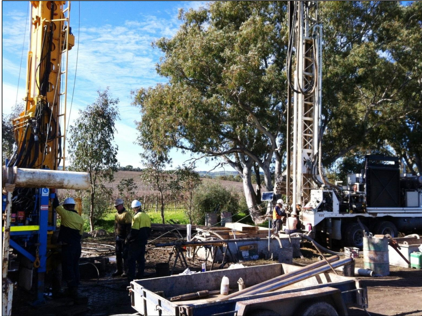
Photo 3: Two drill rigs working at the same time at Site 4. Triple barrel core - rotary diamond drill rig on left for the aquitard coring, and a mud rotary auger on the right for drilling of groundwater bores.
