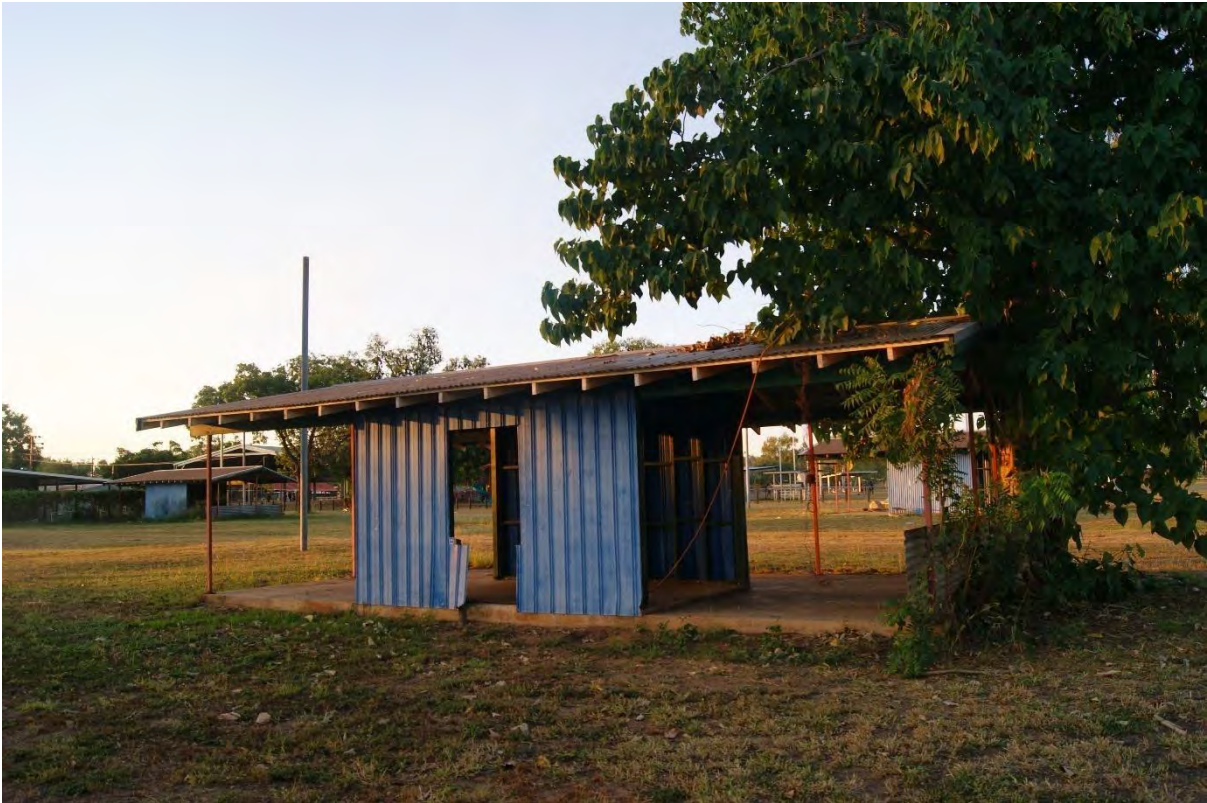
Figure 1.2 Image of Southern aspect of Econo Hut 3 located in situ at Bottom Camp, Barunga (Photograph: Elspeth Hodgins 23/04/2022).
