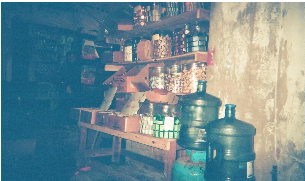
Figure 37: Wall of a shop, showing flaking paint on a damp wall (201, photo 16)
