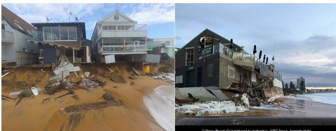
Figure 2.4 Property battered by high tides in Collaroy Beach. Source: Photos by Amanda Hoh, ABC news, 2016
