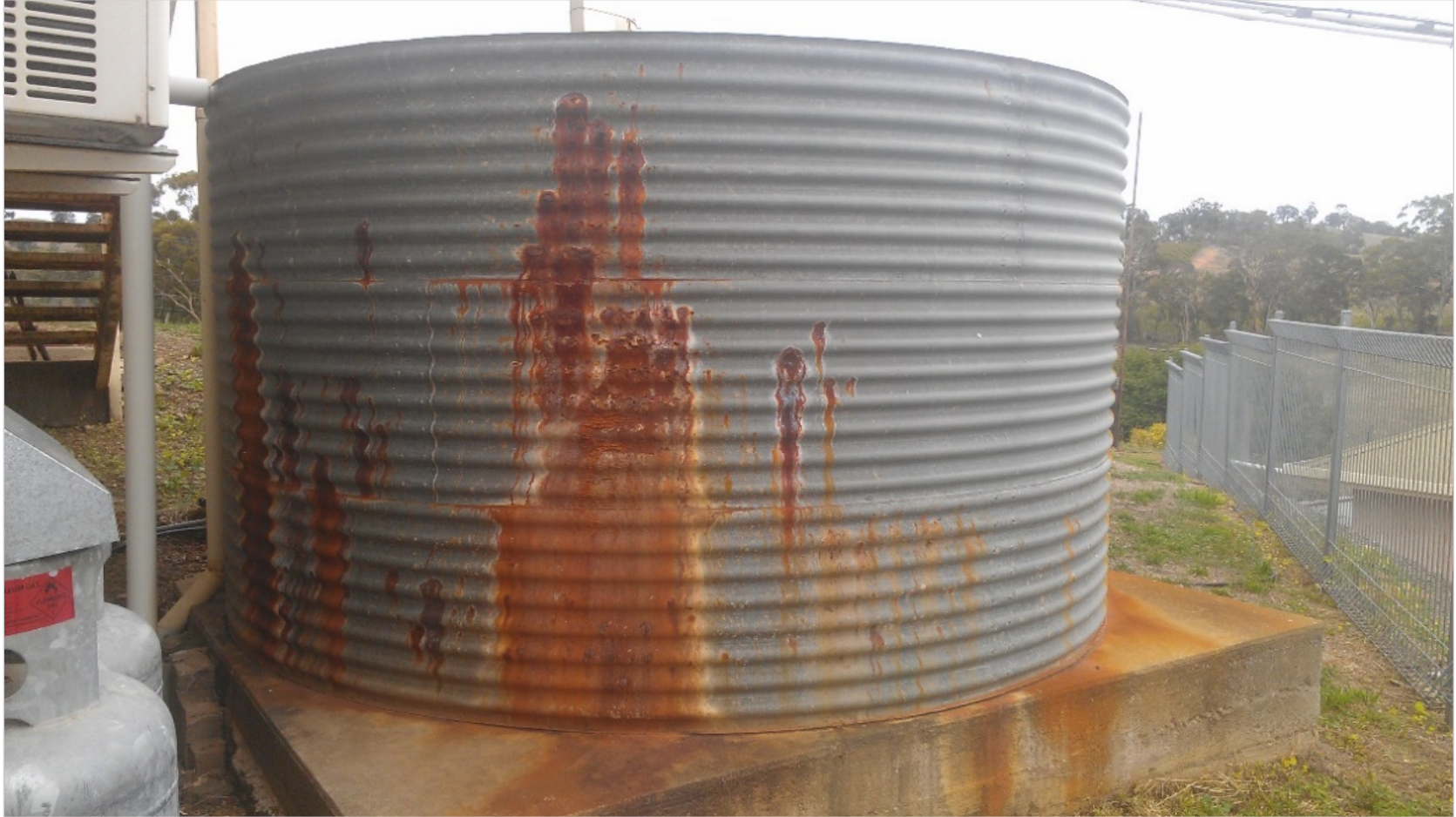
Figure 25. Corrosion on galvanised steel rainwater tank, photo Adelaide Hills, 2016.
