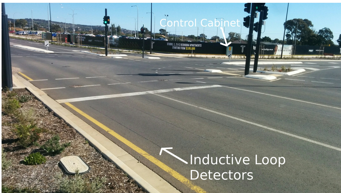
Figure 2.2: Photograph of a typical intersection with loop detectors (foreground) and control cabinet (background)
