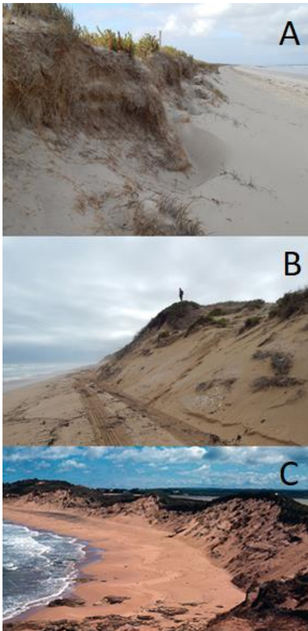
Figure 2: Examples of foredune scarps from (A) small (1m high, with some post-scarp fill and echo dune), (B) moderate (8m high), to (C) large (20m high) (top to bottom). The ability of the foredune to recover and the subsequent stability is generally lower as the scarp height increases.
