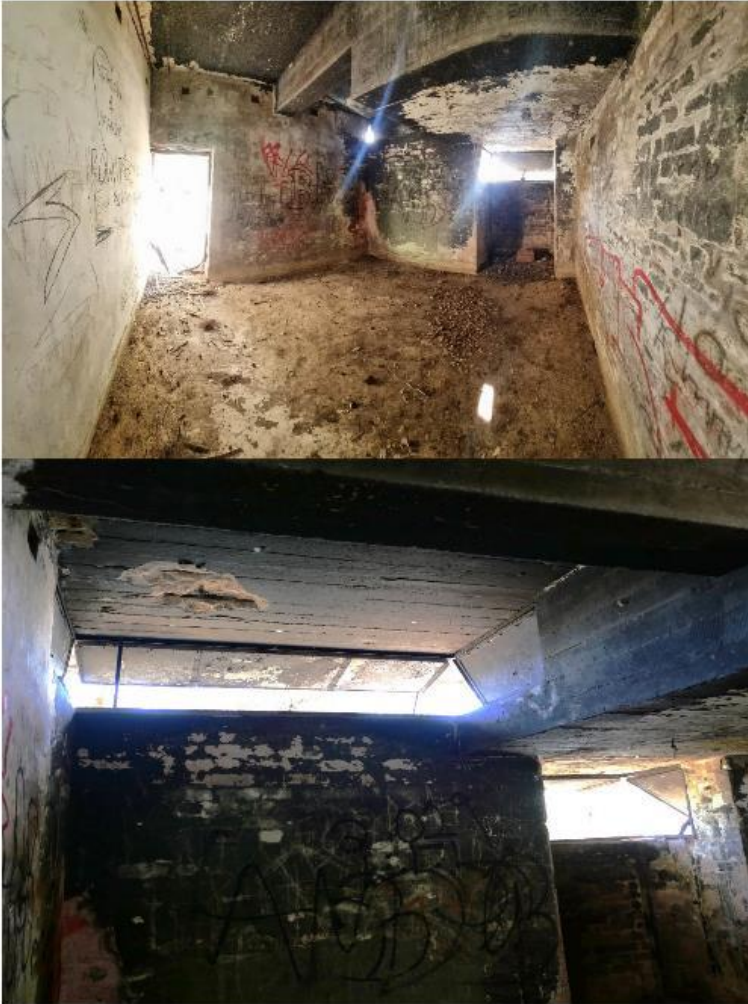
Figure 4-11: Hungry Beach control hut internal. There is a plain concrete floor and evicent brickwork behind the render type walls. The windows are set on two levels, similar to Juno Point though no scar of a mounting structure was evident. The roof is riddled with cancer and rusting reinforcement steel and it is evident that it has been on fire or exposed to fire at least once. Hungry Beach is a public accessible location whereas Juno Point is Government Land where permission is required to enter. The difference in the condition of the sites is this limiting access factor and National Park Service not recognising the significance of Hungry Beach.
