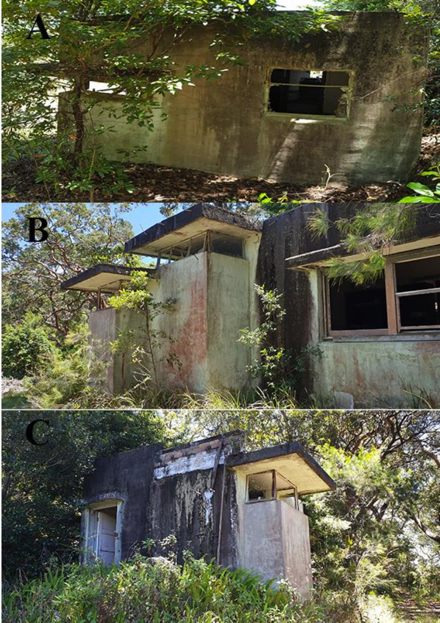
Figure 4-5: Exterior of control hut displaying the state of dis-repair and construction type. A- North wall. B- East wall with observation windows. Evident are the metal rod protrusions for camouflage/blackout curtains. C- South wall with entry door. Exposed brickwork on the roof area.
