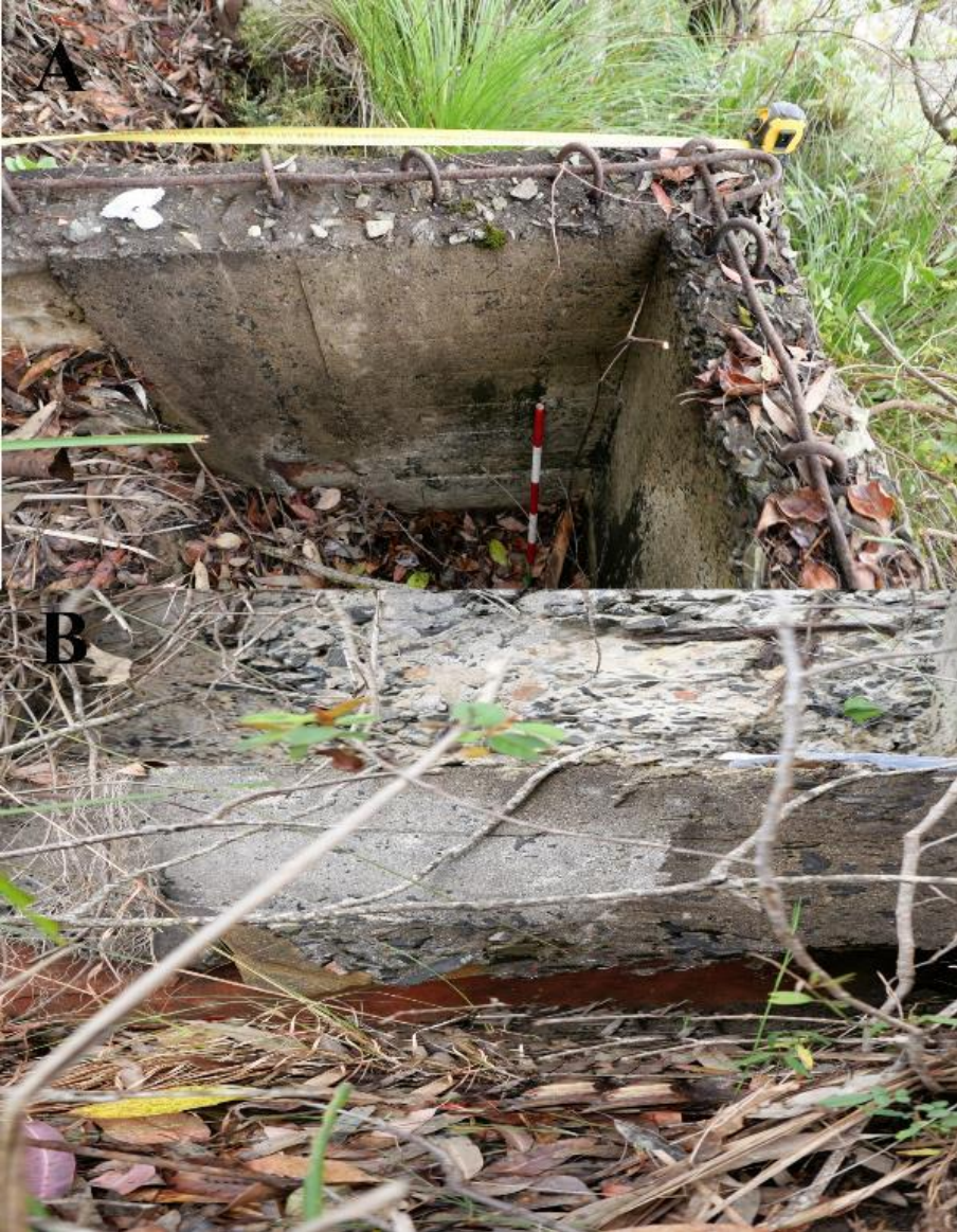
Figure 4-8: Looking into the CASL bunker. A- Showing the depth. Range pole is 10cm increments. Heavy steel loop and wire on the top of a 15cm wide wall. B- Bottom of the outside wall. Red brick supports the concrete wall.
