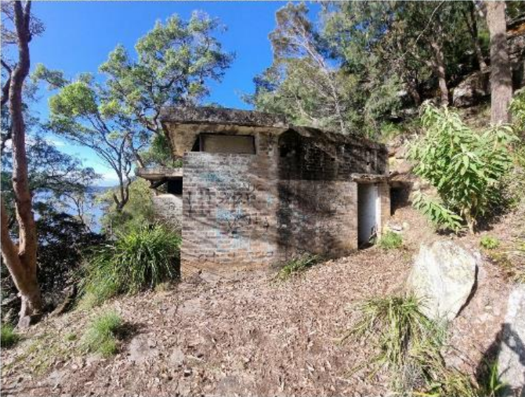
Figure 4-10: External photographs of Hungry Beach control hut. Similar design to Juno Point however does not have an extra room attached. The hut is built up on the side of a cliff using dry walling and concrete foundations are evident on the top photograph. Metal has replaced the glass, this appears to be a recent addition however as with Juno Point they are cantilevered opening outward. The back of the hut is cut into the mountain with the access door having a large concrete lintel over it, though no hinged door is attached.
