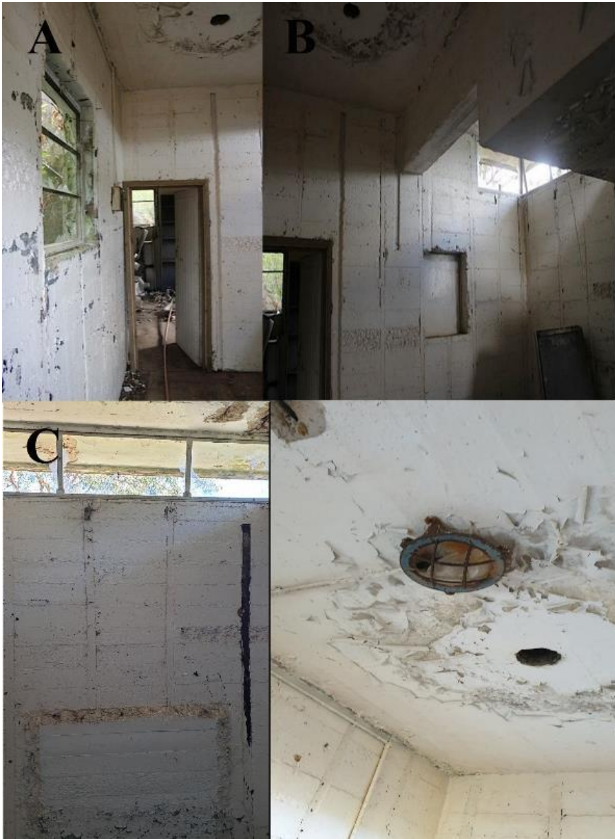
Figure 4-6: Inside the control hut. It is considered all paint is original and hence lead-based. A- Looking north from the entry door through to 2 nd room. The floor is lined with masonite over the original floorboards; the construction method is evident with the negative of the original framework when concrete was poured. B- Looking northeast, showing a 'pass through' window now blocked. C- Upper observation window and the scar of an observation platform. It is likely used to mount ranging optics. D- Original light fixture. Also evident is some concrete cancer and rusting reinforcement. The round hole in the roof extends to the outside, and further investigation into its use is needed.
