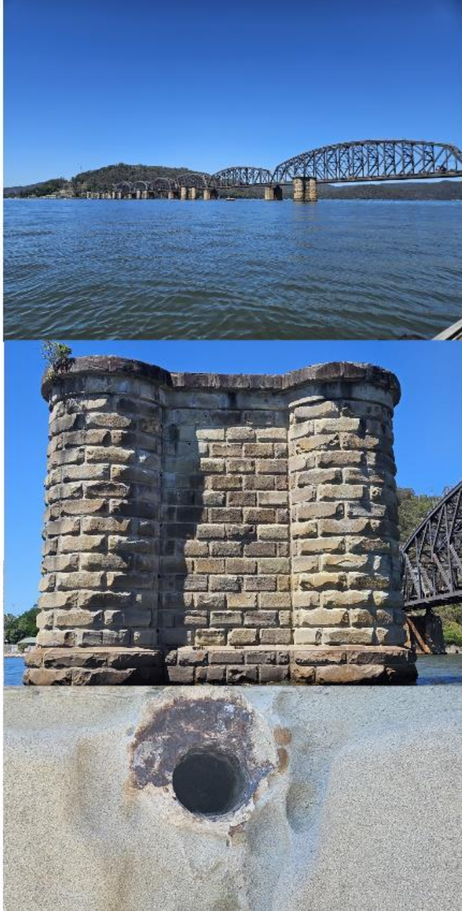
Figure 4-23: The span of the old Hawkesbury River Railway Bridge front of new bridge (top), photograph of a single pylon that has six holes drilled between the round and flat sections with random holes drilled in the face of the flat section (middle). Clos up of a hole drilled in flat sections of the pylons (bottom). Hole diameter 100mm, depth unknown.
