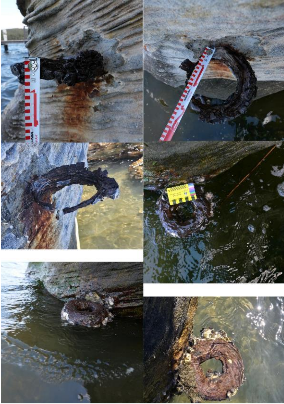
Figure 4-18: Close up of the securing rings. Upper ring (1-3) shows extensive corrosion and laminating, it is not affected by tidal movement since it is 1m above the bottom ring. Bottom ring (4-6) still remains in near original form, though some
