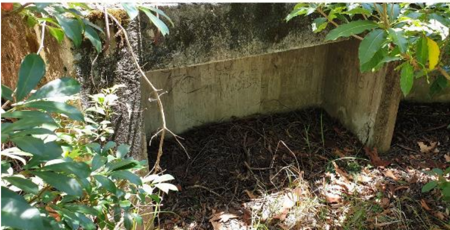
Figure 4-30: Example of graffiti in the ammunition bunker at Juno Point. Further study into the area around the isolated graffiti in a protected area might shed light on the people/students who left their mark for the future.
